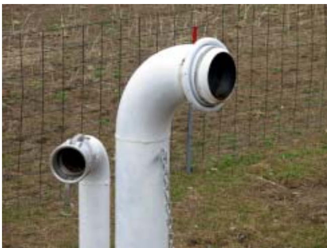
Figure 3. The 6" suction pipes have irrigation pipe connections while the 2-1/2" suction pipes are equipped with camlock connections to save connection time.
