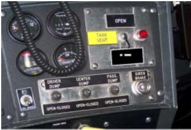
Figure 13. The in-cab controls for the tank vent and the three dump valves are normally used for dump & run operations.
