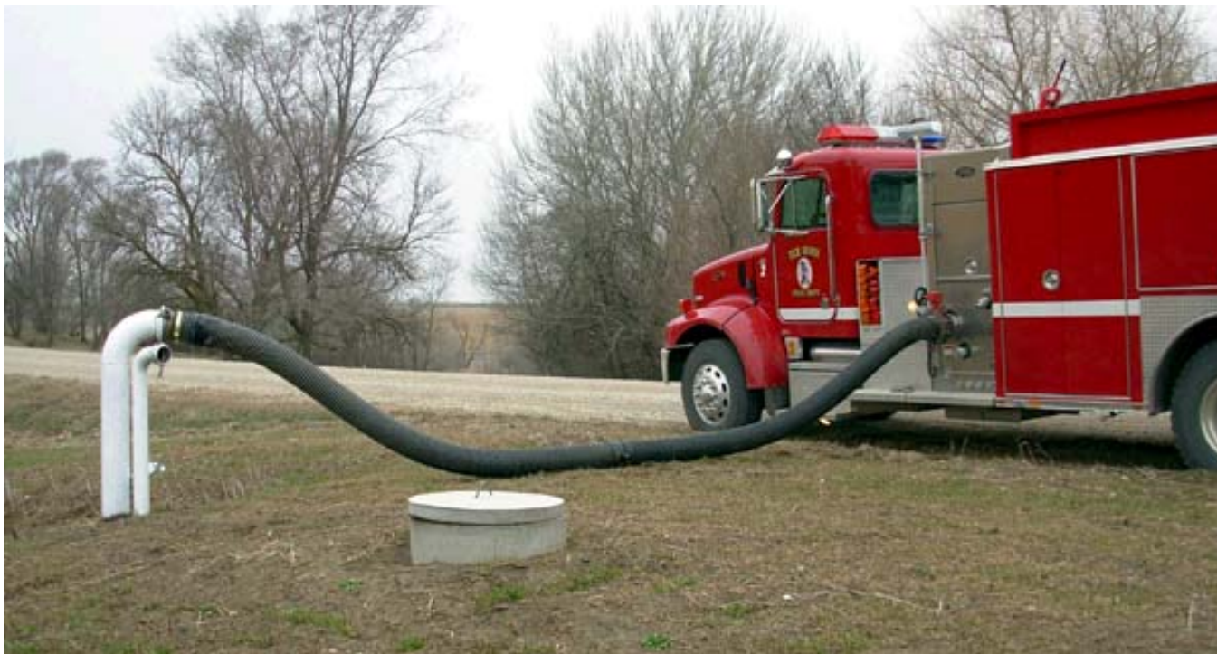
Figure 1. An Elk Horn engine drafts from a suction pipe installed into one of the ten underground water storage tanks they have had installed throughout their service area. Each tank holds between 6,000 and 15,000 gallons and is equipped with a large access opening and a 6" suction pipe for pumper drafting and 2-1/2" suction pipe to allow for portable pump drafting.
